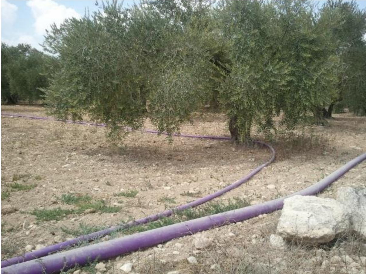
Photo 3.5: Water treatment line for irrigation in Anza
